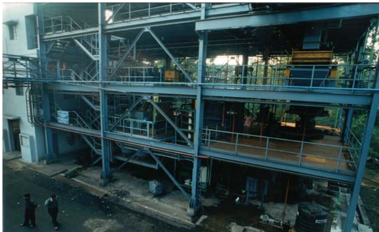
Fine Coal Treatment Pilot Plant
